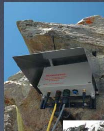
Base station mounted under a combined sun/rain hood
